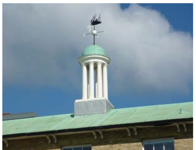
Copper roof and attractive central cupola with feature weather vane, Bowling Green House
