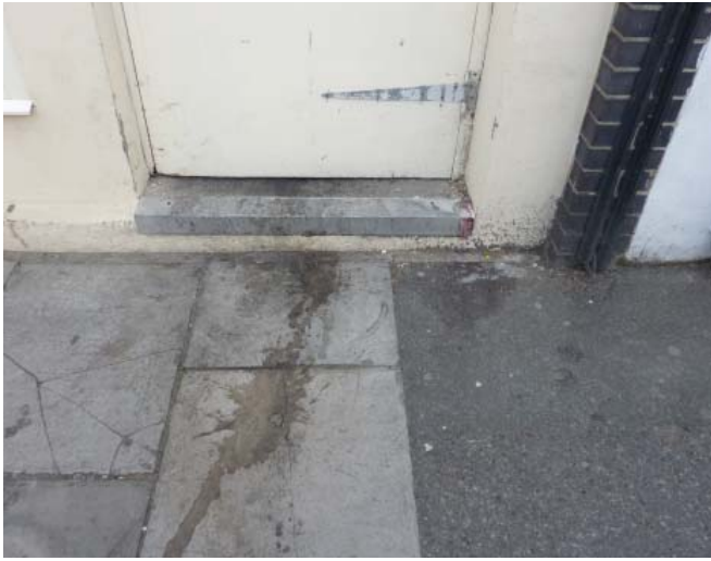
Grease marks left on the paving outside commercial premises, Oxford Street
